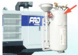
Water tank for water injection system
